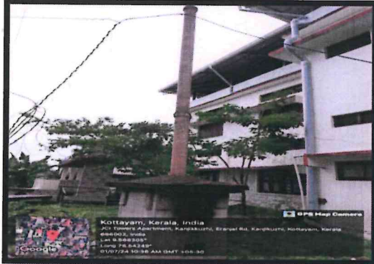
Waste Burning Incinerator
